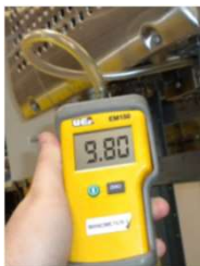
Verify Inlet Pressure
